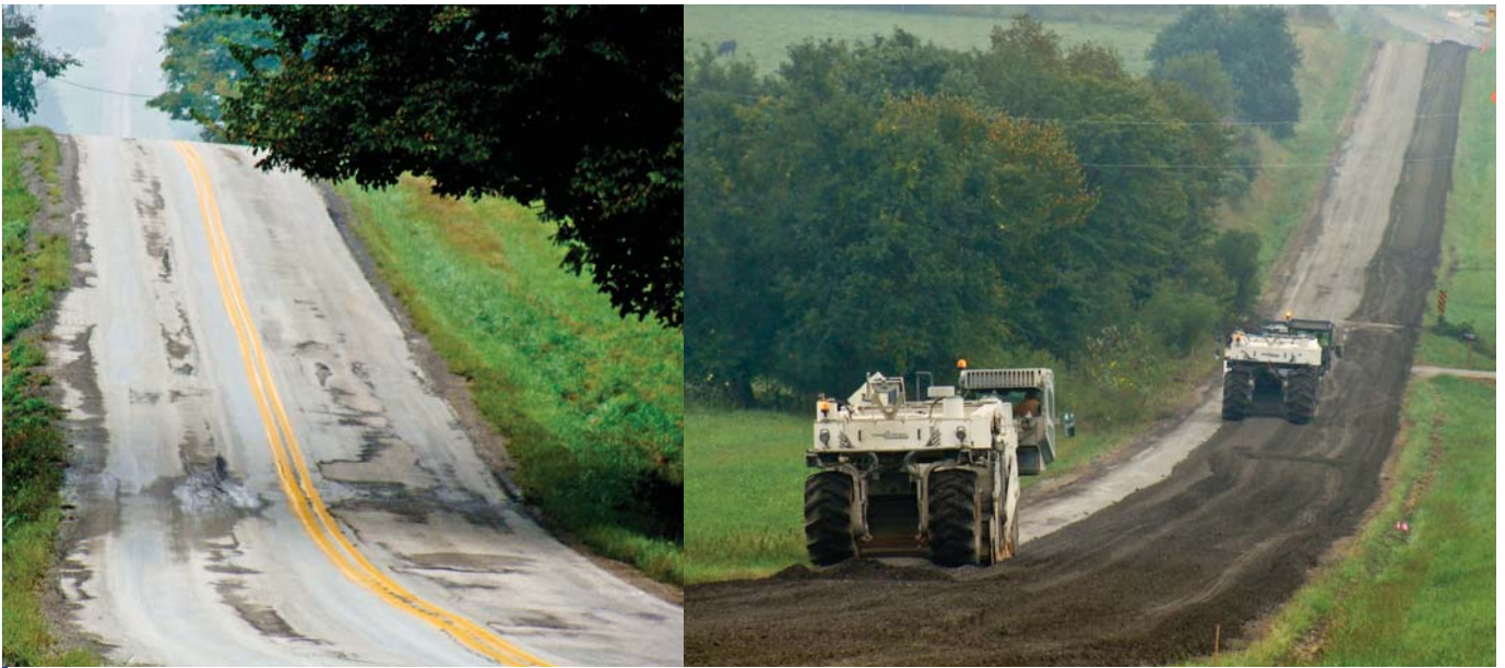
The aggregate base course on Rte. Y that preceded the asphalt pavement had virtually vanished, a victim of years of subgrade pumpings and settlements. Mt. Carmel used two Wirtgen WR 2400 reclaimers for pulverization and mixing.
