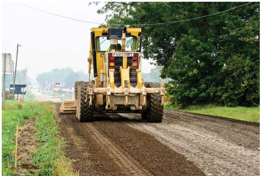
Following pulverization, the section is compacted and graded to a consistent 22-ft width and 2% cross slope. Proper geometry is something that this road has not had in a long time.
